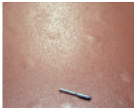
Blisters before Failure
