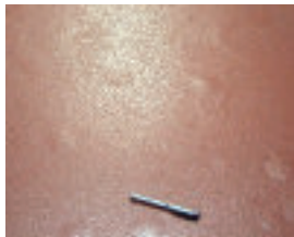
Blisters before Failure
